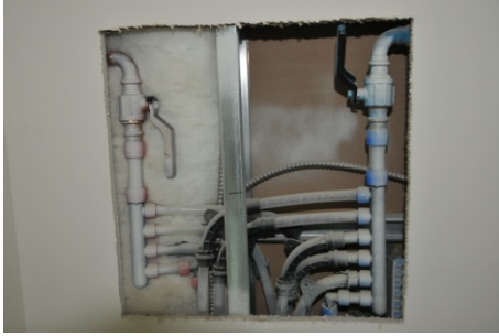
Main (Generally located in a storage room or closet)
